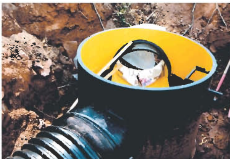
At the returning point, manhole with entrance and exit, pipe inside dike and ladder applied.
